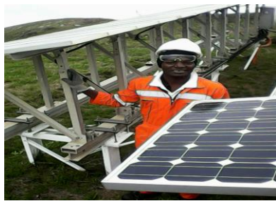
PV SYSTEM FOR TELECOMMUNICATION POLE
